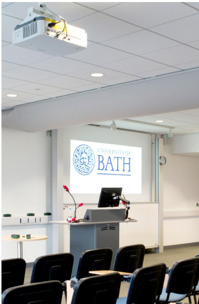
P502HL Laser projector installed across teaching areas at the University of Bath, United Kingdom
